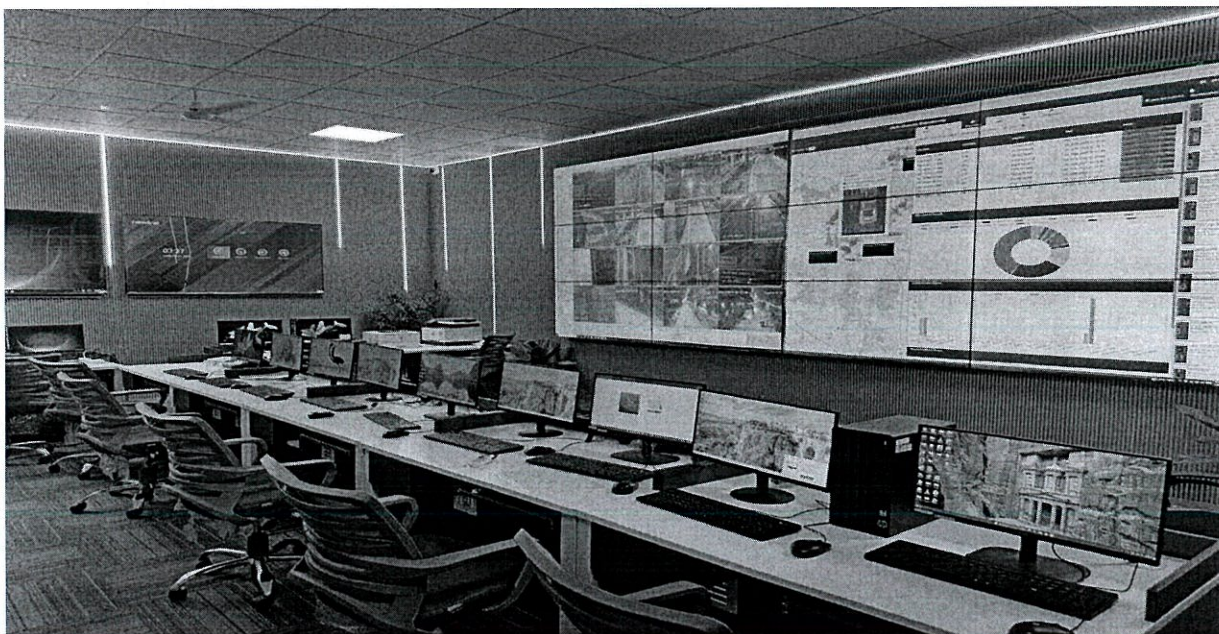
Figure 1: ATMS Control Center - Dwarka Expressway
